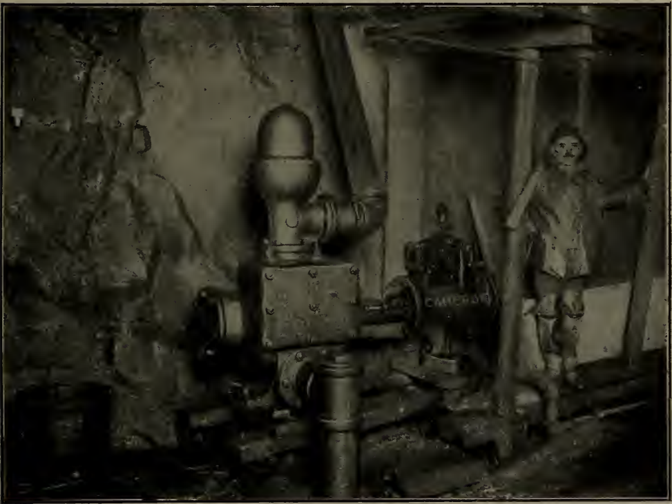
Photograph taken in Pennsylvania and Long Island R. R. Tunnel. Cameron Station Pump handling the drainage water, which seeps through the rock and earth that separate the tunnel from the river bottom.
